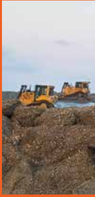
FOLLY BEACH 2.0 Beach renourishment is a vital project to battle beach erosion
